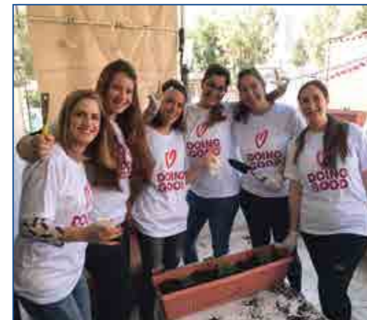
AIG employees renovating and gardening "Alma" as part of Good Deeds Day
